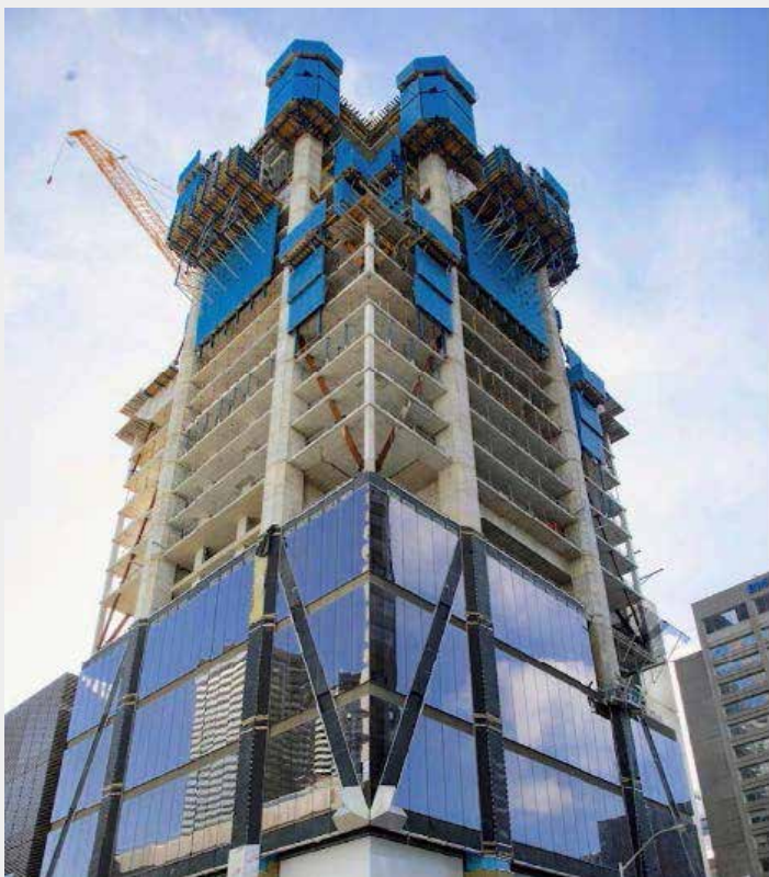
Fig. 17: Exterior view of the tower early in construction showing the ACS at the top, hanger columns and envelope progress above the ground floor retail. The RCS system was not yet installed in this photo
