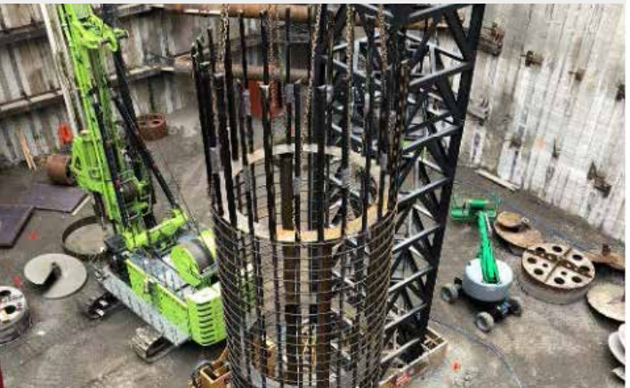
Fig. 13: Caisson is ready to be installed from the base of excavation into the lined shaft to the rock
